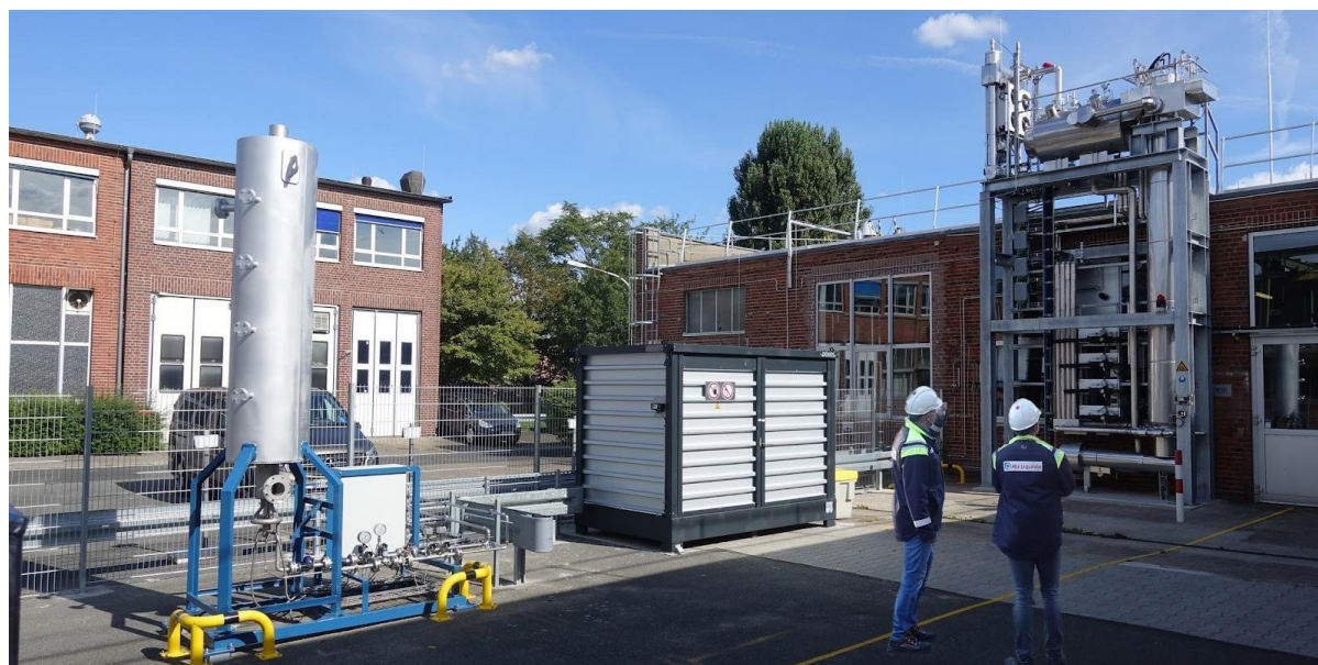
Figure 1: Multi-stage methanol pilot plant at Air Liquide Innovation Campus Frankfurt
