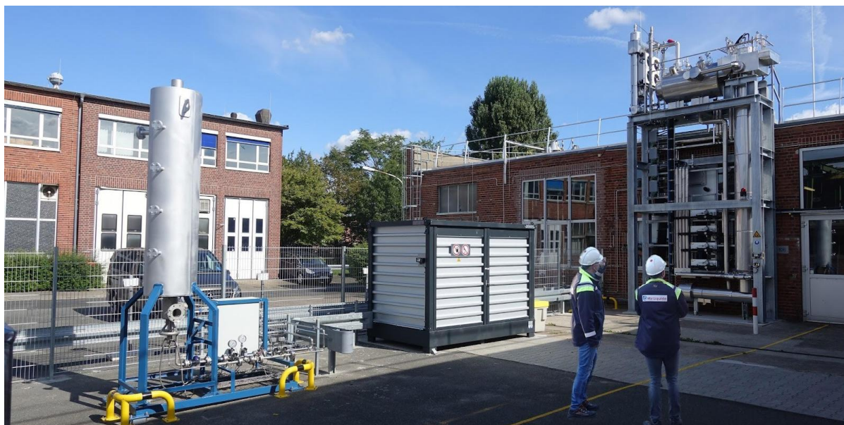
Figure 1.1: Multi-stage methanol pilot plant at Air Liquide Innovation Campus Frankfurt
