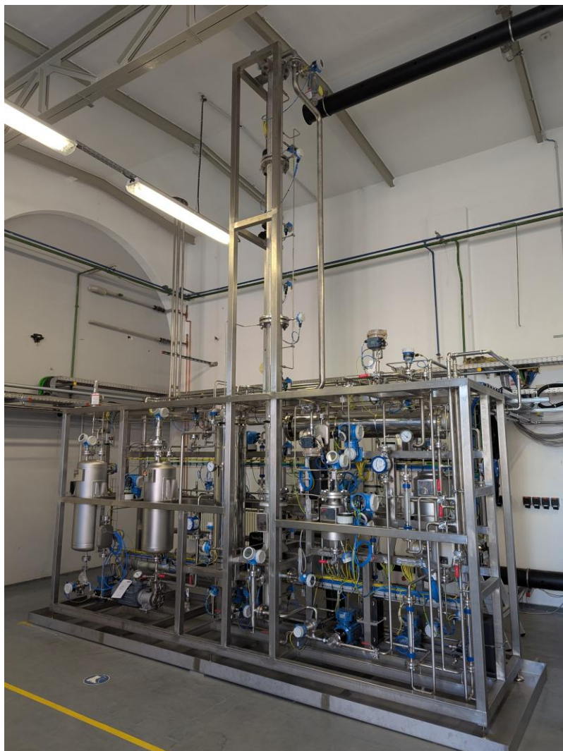
Figure 2.1: New distillation pilot plant at Air Liquide Innovation Campus Frankfurt
